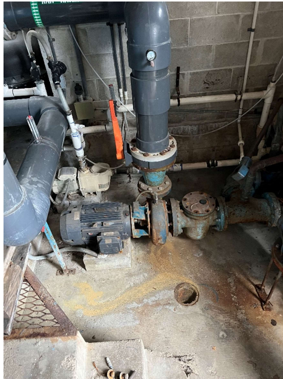
Main Pool Recirculation Pump Assembly
