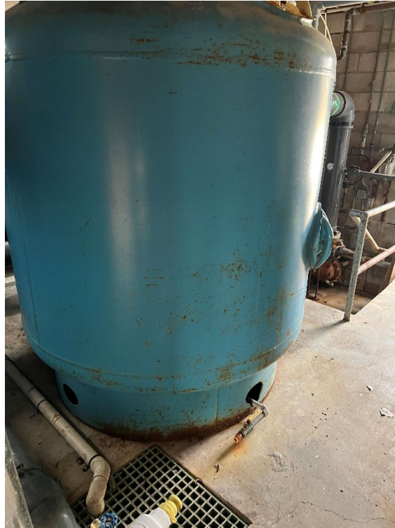
One of Two High Rate Sand Filters (Main Pool)
